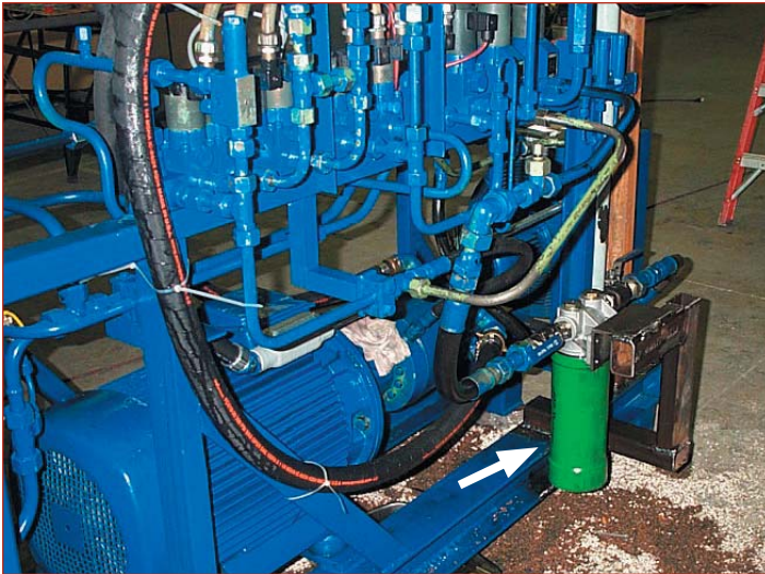
FilterMaster ADD-Vantage 9000 – equipped with a 25 micron, stainless steel, reusable oil filter and secondary magnetic filtration rod – on a Wemhoner press. (Filter indicated by arrow)
